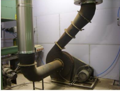
Induced Draft Fan
